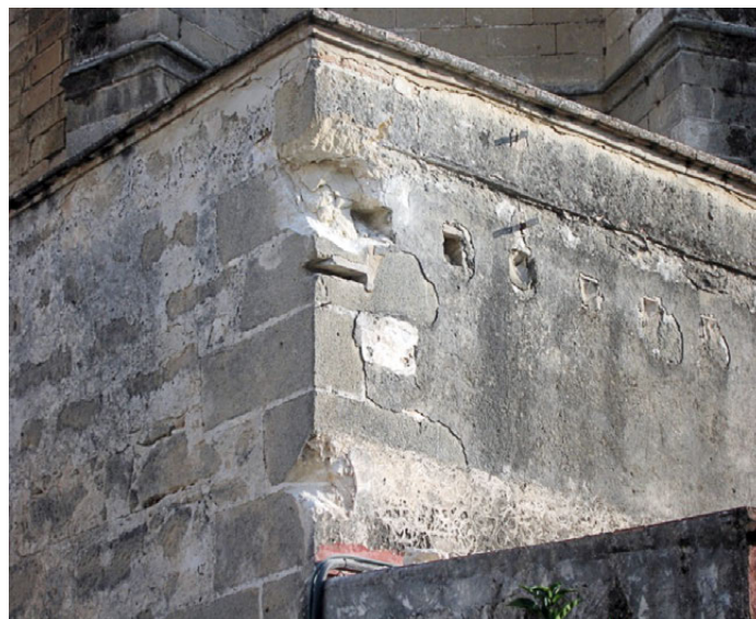
Figure 3. Marks on building wall
