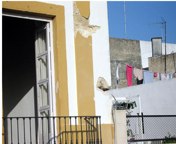
Figure 4. Marks on building wall
