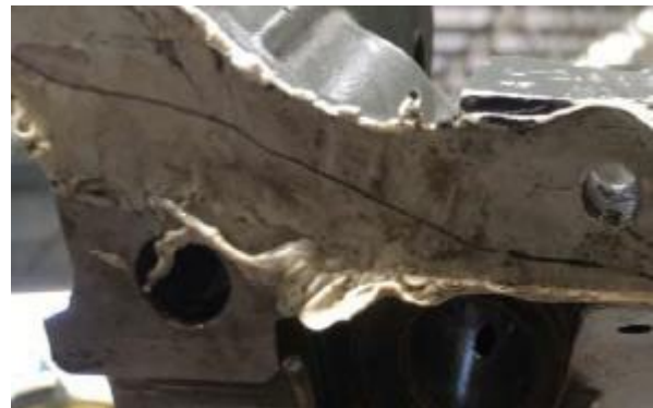
Photograph 34. Silicone in the joint of the semi-sump
