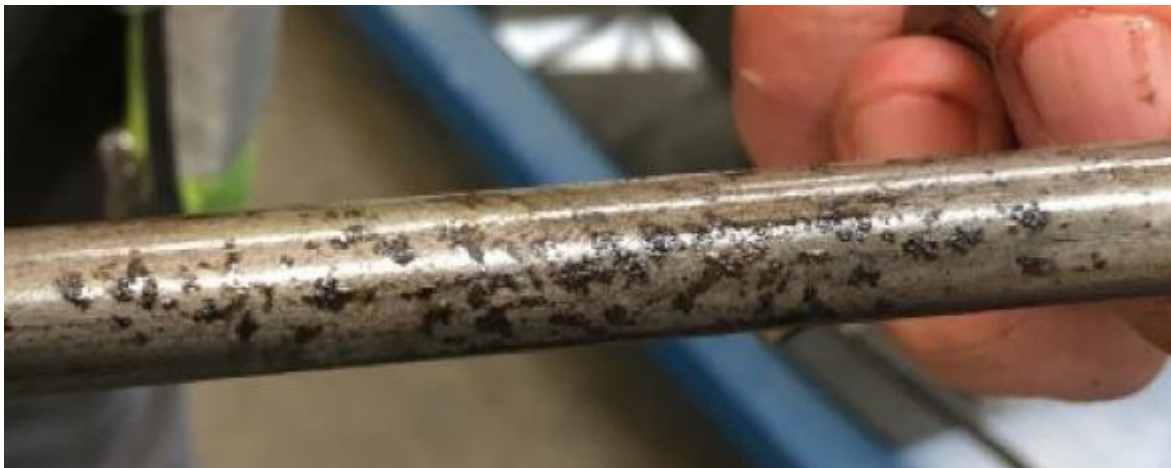
Photograph 25. Presence of oxidation in the valve rod
