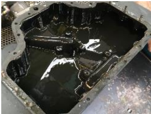
Photograph 27. Oil in the oil sump
