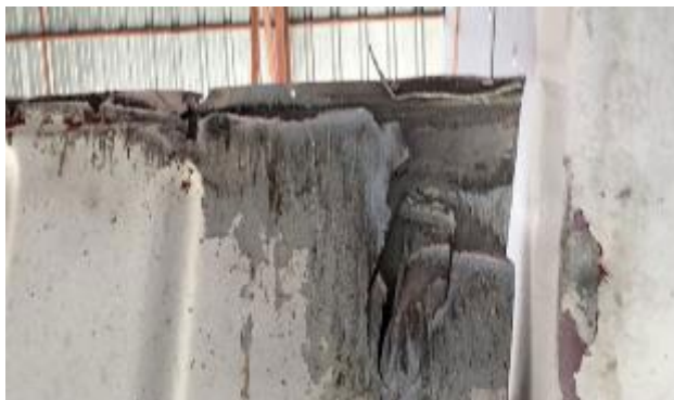
Photograph 11. Damage to the left flap
