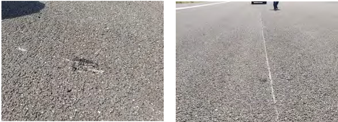
Photograph 4. Marks on the runway
