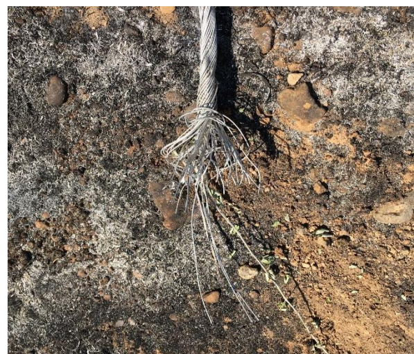
Photograph 18. End of the severed cable from the southern slope
