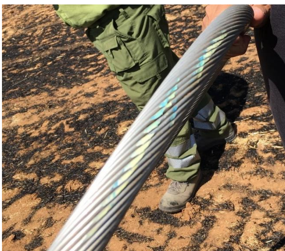
Photograph 17. Colour transferred to the cable by the impact
