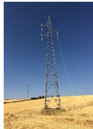
Photograph 16. Pylon and severed cable from the incident
