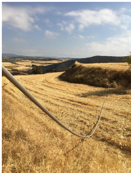
Photograph 19. Severed cable from the northern slope
