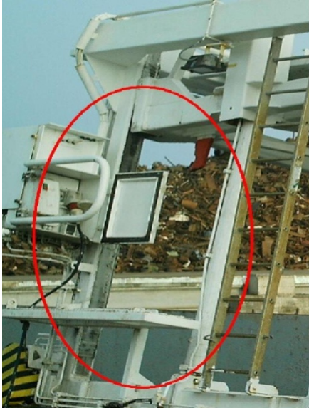
Photo 8: Limited anti-fall protection on the operating platform with an 'open' door (see also photo 3).
