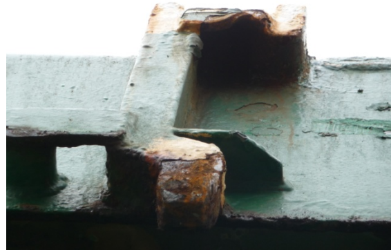
Photo 9: Damaged attachment point of the fallen hatch.
