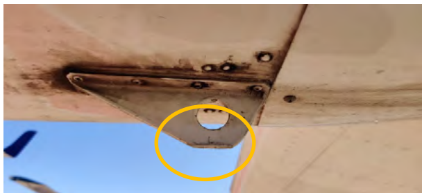
Photograph 7: Tie-down bracket on underside of tail
