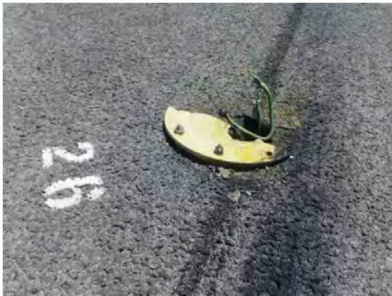
Photograph 22: Runway edge light remains
