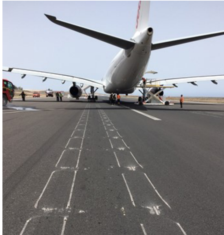
Figure 11. Marks left on pavement
