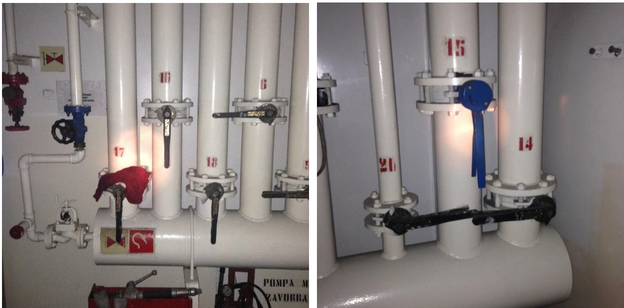
Photo 4: State of Drencher valves.
