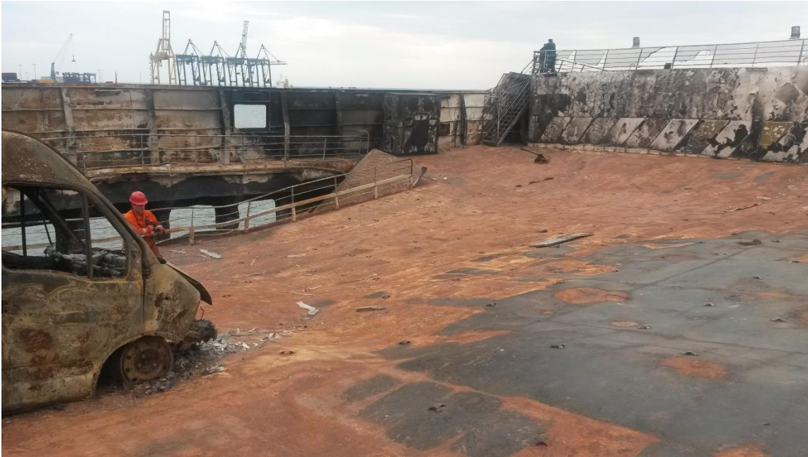
Photo 5: View of the collapsed area
