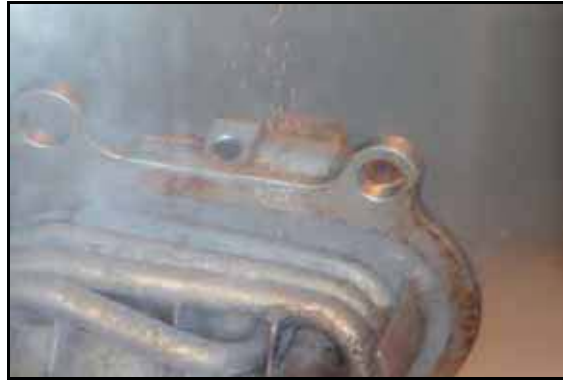
Photo No. 4: Sensing tube leak
