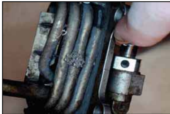
Photo No. 5: Sensing tube leak
